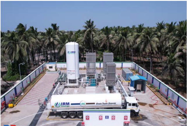
L-CNG Station for IRM Energy at Gujarat
