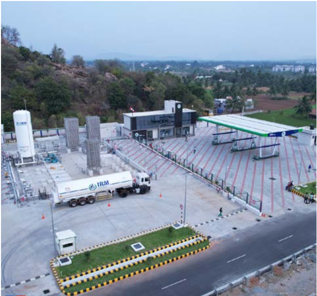
LCNG Fueling Station
