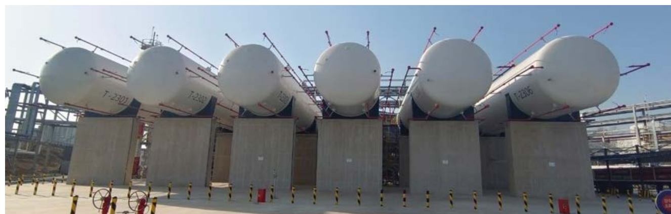
Liquid Hydrogen Tanks
