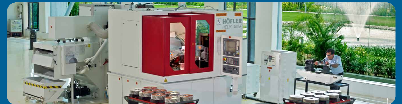
Inside view of BMCE Plant
